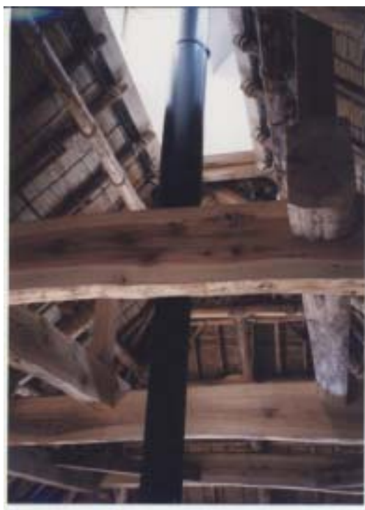
Figure 4 The beams which remain the traces of mold and the top light well with reflection boards.
